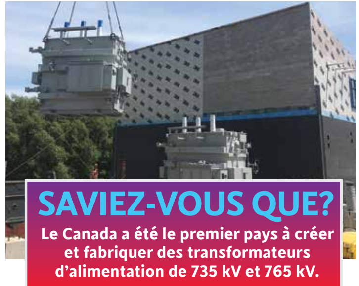
Photo courtesy of Northern Transformer
