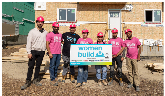
Schneider Electric, Calgary, AB - October 7, 2025
